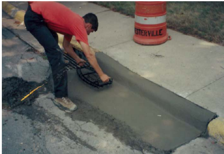
Figure 11. A Westerville employee stamps the message: “No Dumping, Flows to Creek” into fresh concrete near a storm drain (Photo source: City of Westerville, 1998)
