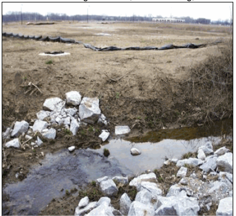
Figure 9. A failed sediment fence beside a large plot of land undergoing development allows runoff of silt into a tributary to Alum Creek. Photo source: Alum Creek and Tributaries Watershed Action Plan, 2005.
