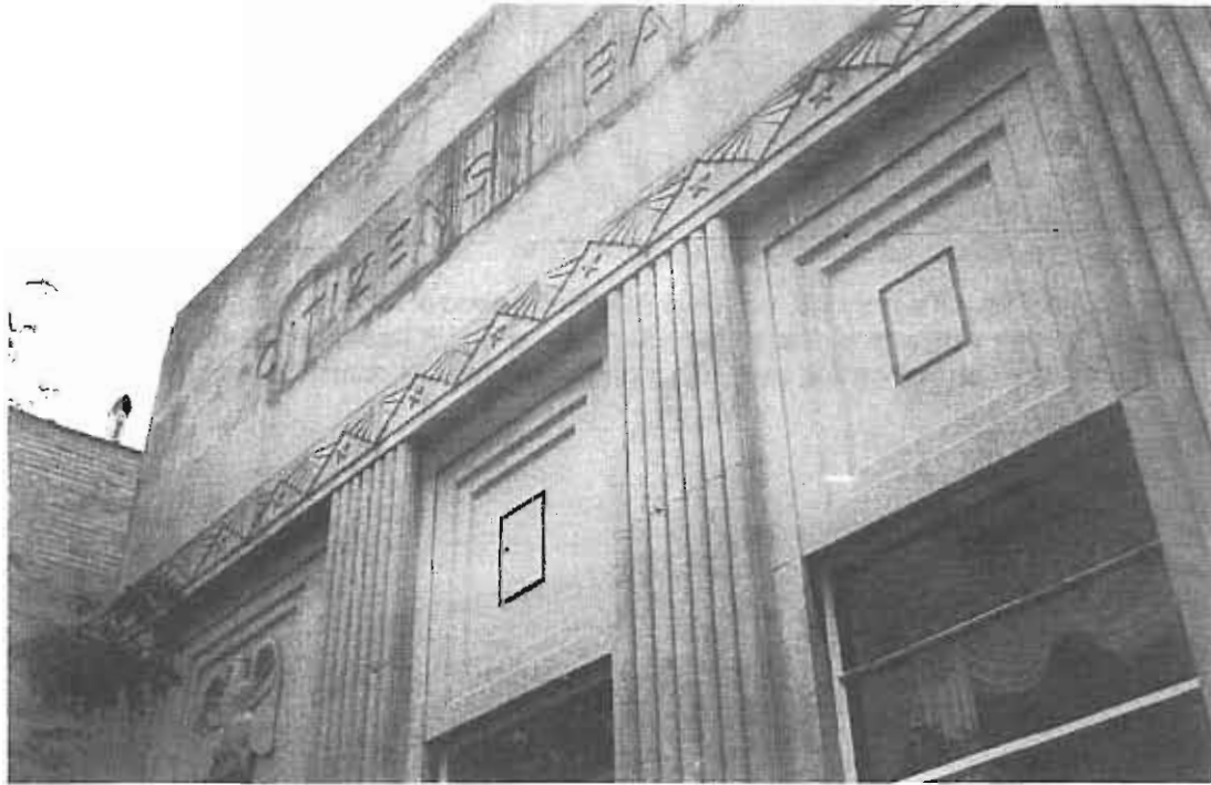
By the 1920s and 1930s, many buildings had parapet walls with little or no ornamental treatment. This Uptown bank is an excellent example.
