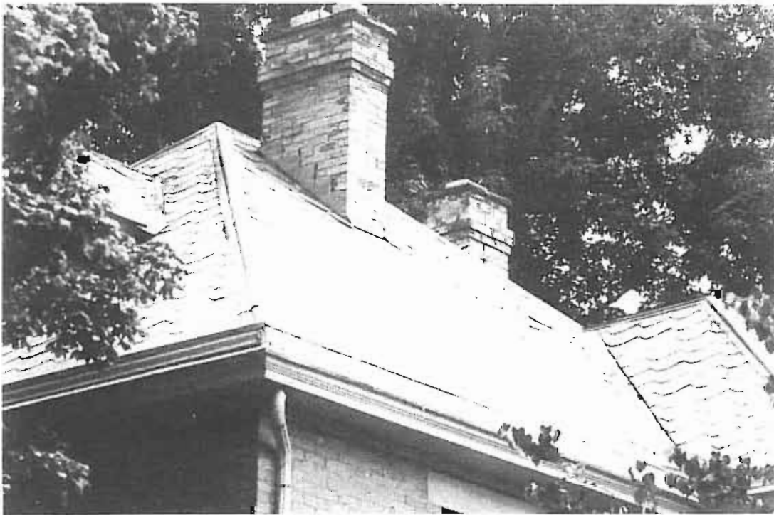
This is a typical late 19th or early 20th century roof, in this case covered with shaped slate shingles, with all its waterproofing elements intact: capped ridges, flashing at chimneys and in valleys, and a system of gutters and downspouts. These are "box" gutters, which are built into the roof structure above the eaves.
