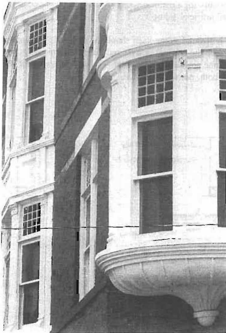
The Holmes Hotel combines both wood and sheet metal elements to create a varied and interesting design. Both materials should be kept well painted.
