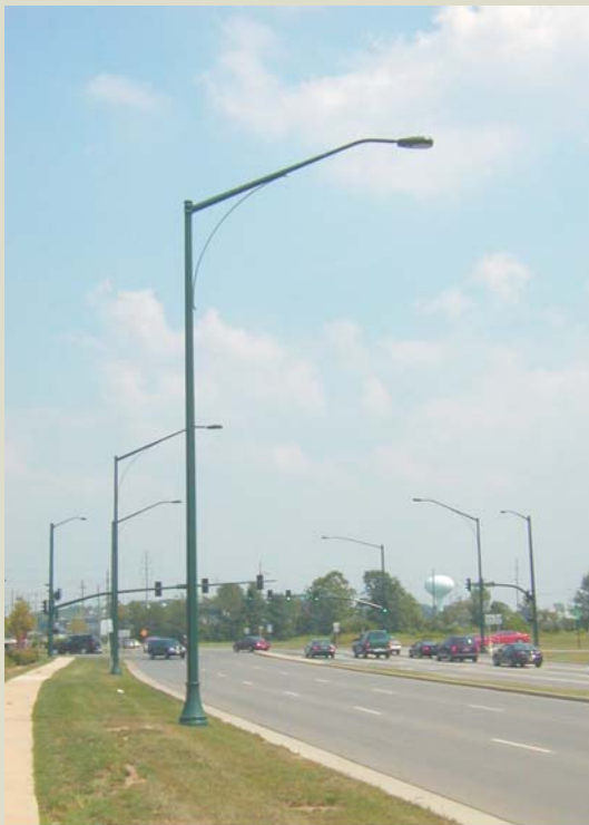
Recommended light fixture for Gateway and State and Schrock Districts
